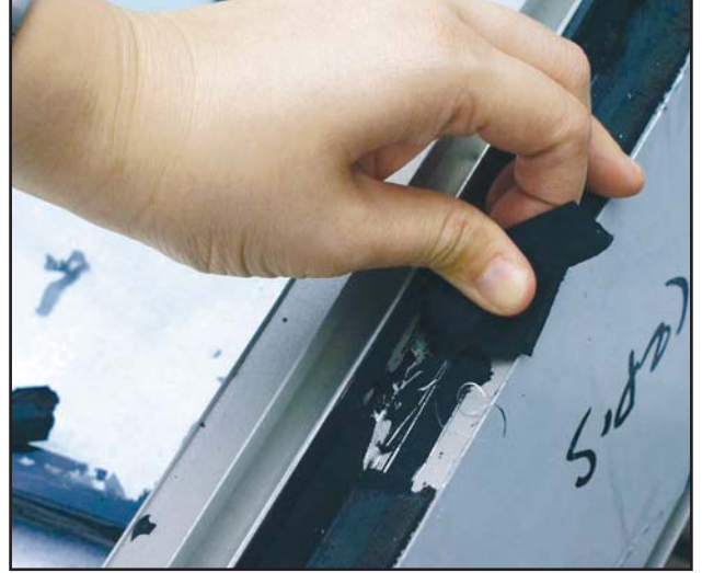
Picture 18: Adhesive failure, deglazing test negative
